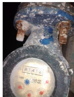
Meteran Outlet IPAL
